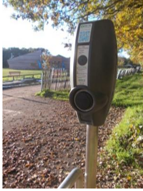
ELECTRIC VEHICLE CHARGING POINT
